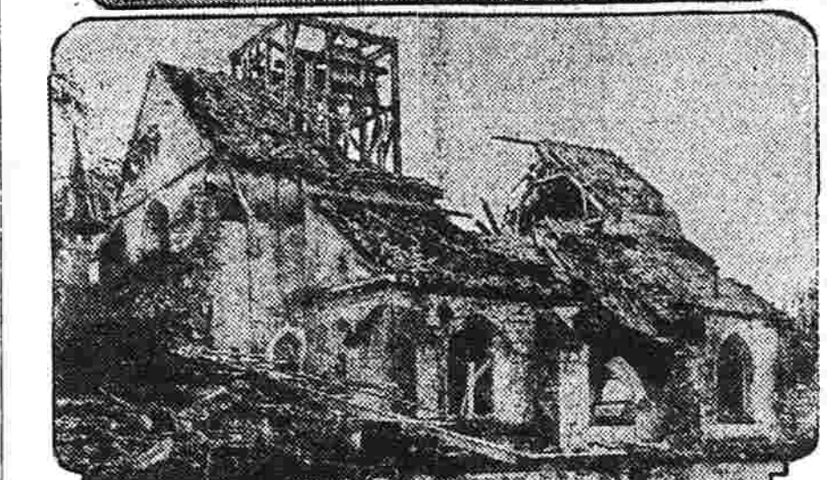
When the Twenty-Sixth Division captured Belleau in July, 1918, after their artillery fire had reduced the village to ruins, the 13th century church was wrecked as shown in the lower photo. But the men of the same division rebuilt the structure, and it is shown above nearly completed. The rebuilt church was dedicated October 10 and Col. Harry Bissell of this town was present when the ceremonies took place.
